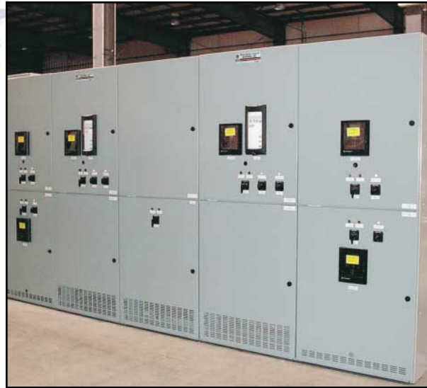
Main-Tie-Main Switchgear With Solid State Protective Relays
