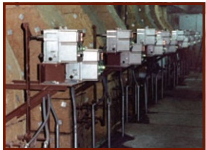
Jordan SM1700 electric actuators control over-fired air dampers.
