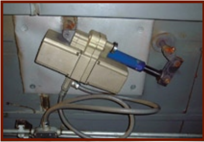
A Jordan LA2000 modulating electric linear actuator operates a secondary damper.
