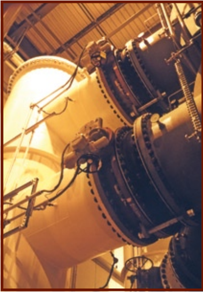
Rotork IQ electric actuators operate 48-inch butterfly valves located about 20 feet above floor level.
